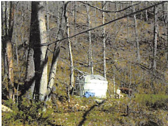
Collection Tank at base of hill
